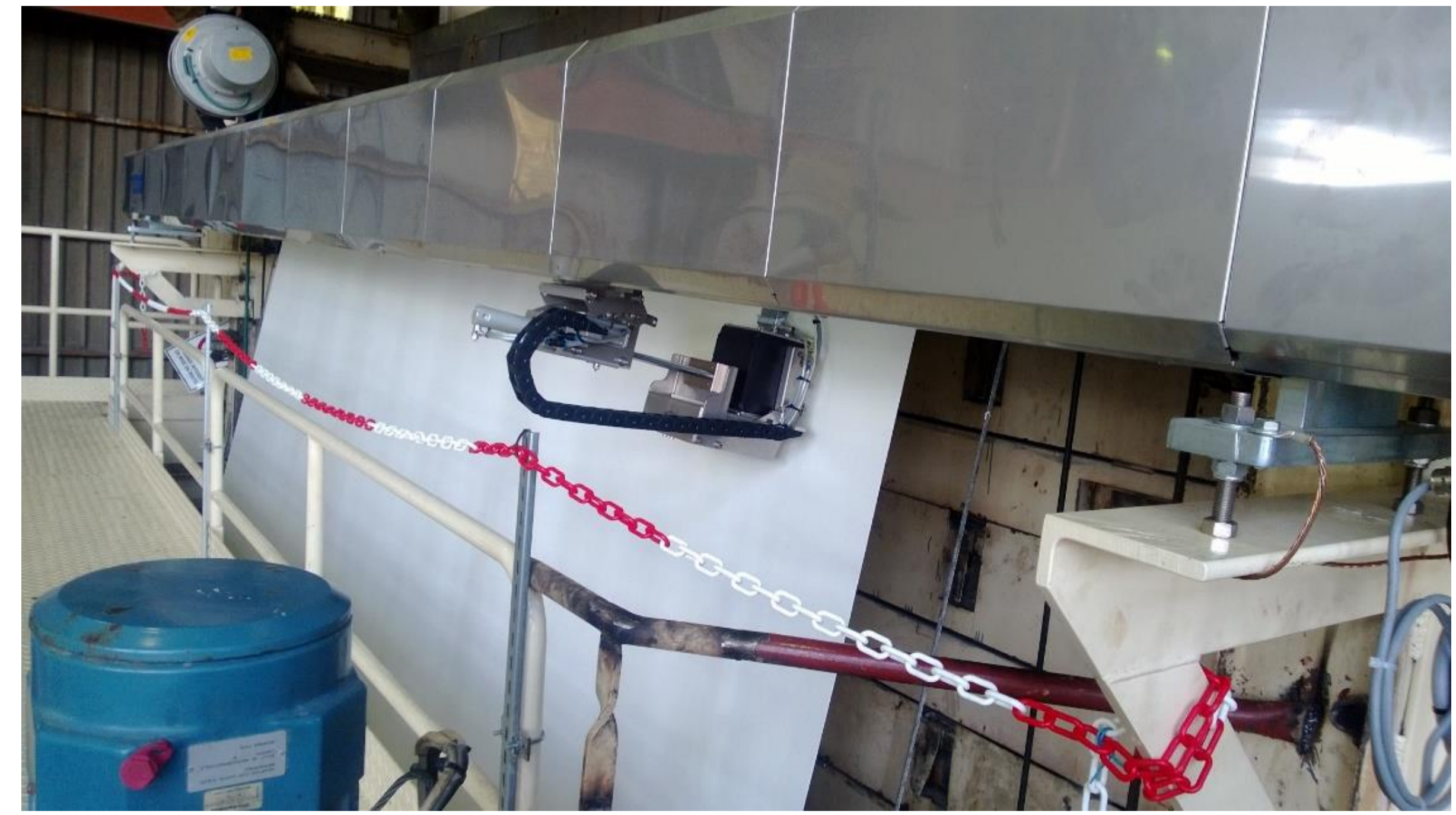
Pulp Dryer line installation before dryer using single-sided scanner and Microwave Sensor
